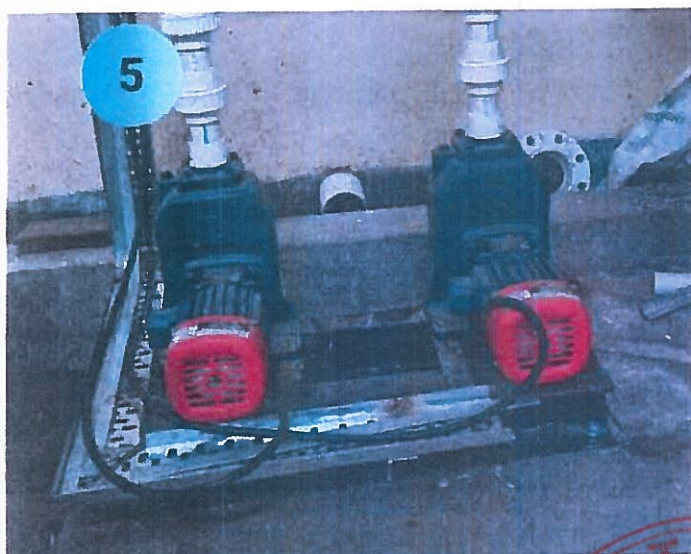
Sludge Recycling Pump
